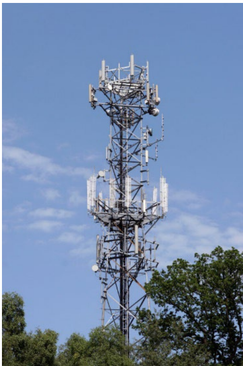
Figure 3.2: Example of a ground-based tower [Source: Analysys Mason, 2023]
